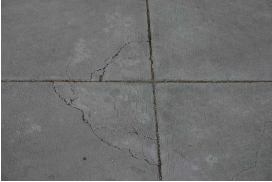
Photograph D Largest Crack in Palm Springs Library Parking Lot
