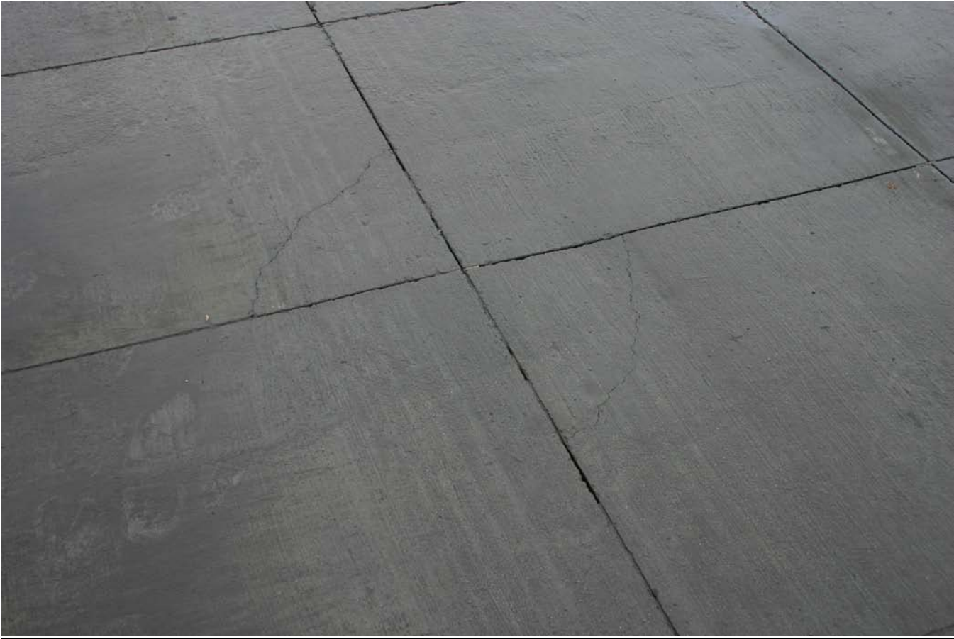
Photograph F Alamo Truck Stop – Corner breaks in UTW in portion extending from scale
