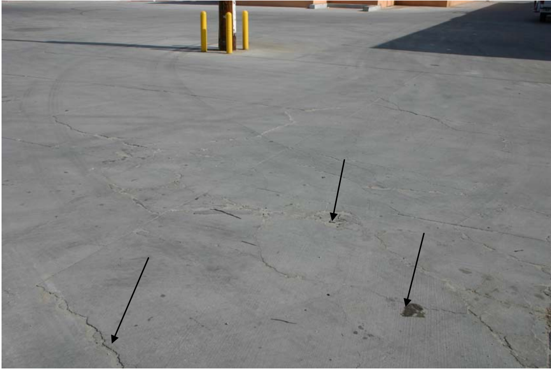
Photograph B Indio Heights Center – Cracking at truck unloading/loading area
